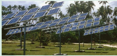
Figure 12.5 Solar panels on Nukubati Island
