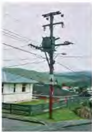
Figure 24.3 Transformers produced in many shapes and sizes.
