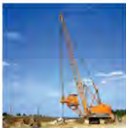
Figure 6.10 When the float falls, it gains kinetic energy and drives the pile into the ground.
