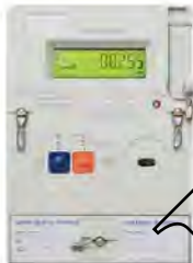
Figure 6.14 A domestic electricity meter.
