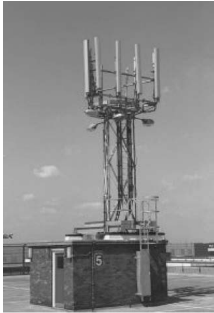
FIGURE 3.5 Typical GSM radio site.
